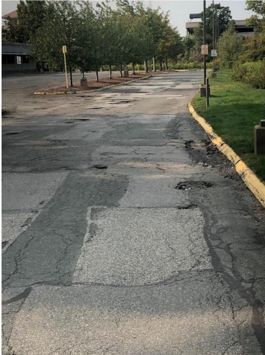
Dangerous condition of Parkway approaching 100Q
