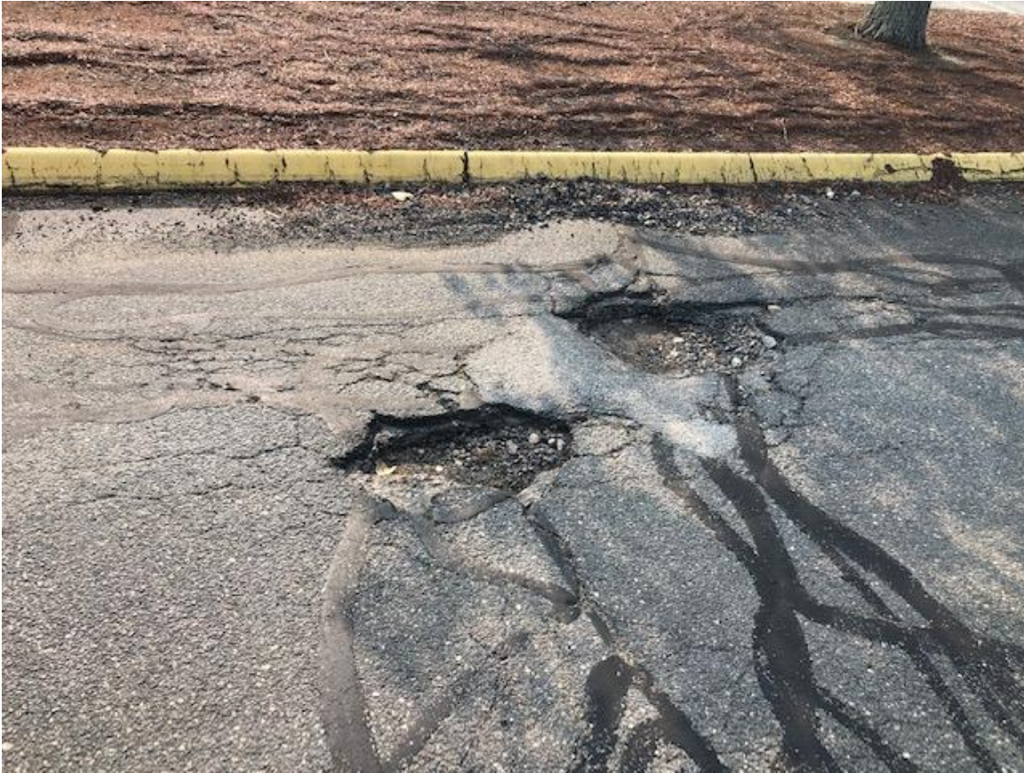
Typical Potholes and broken up pavement of Parkway against curb at 200Q
