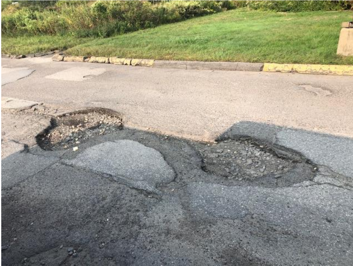
Potholes and disrepair in Parkway at 200Q
