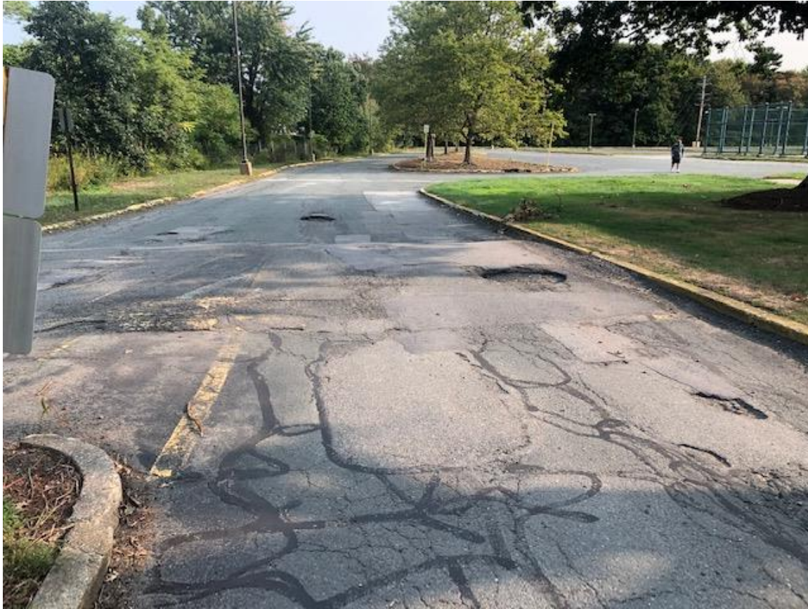
Parkway Potholes and broken pavement in front of 200Q
