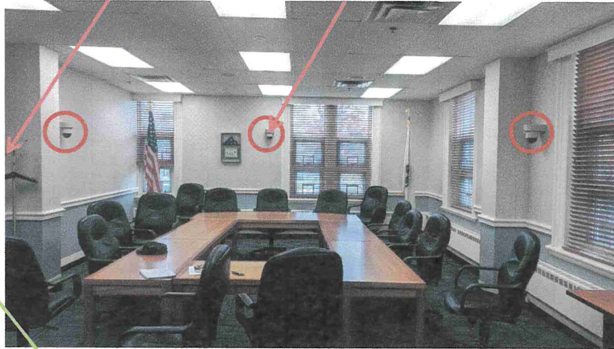
Equipment Racks Panasonic SD 954 PTZs (2004)
